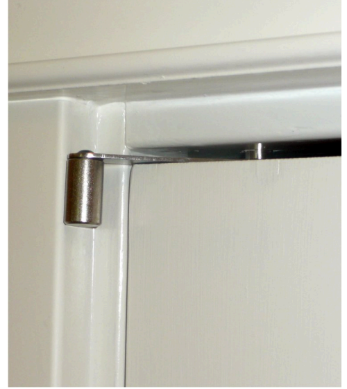
6. IF THE GAP BETWEEN THE DOOR AND JAMB IS LARGE, ADJUST THE POSITION OF THE DEADBOLT DOWN TO THE TOP EDGE OF THE DOOR AS SHOWN. LEAVE JUST ENOUGH GAP SO THE DEADBOLT DOES NOT RUB THE DOOR WHEN IT IS OPENED AND CLOSED. (KEEPING A MINIMAL GAP BETWEEN THE DEADBOLT AND THE TOP OF THE DOOR GREATLY IMPROVES THE STRENGTH AND ABILITY OF THE DEADBOLT TO RESIST FORCED ENTRY).
